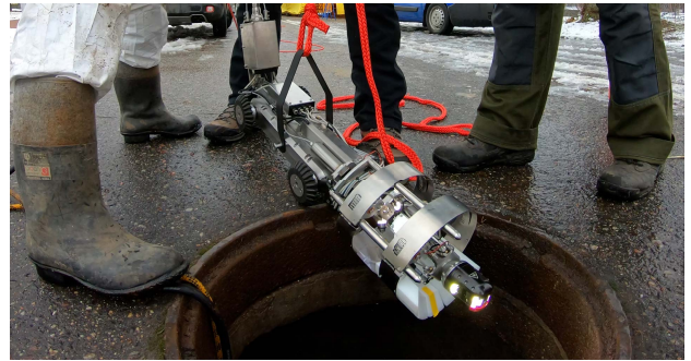
(b) Two micromole devices being installed by a robot in a DN250 pipe through a manhole in Legionowo, Poland, on February 2019.
