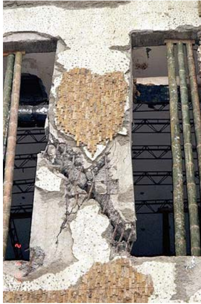
Figure 4-15: Bidiagonal Shear Cracks and Spalling (Shear and Compression Failure) Alejandro Asfura/EQE International, Armenia 1999;
