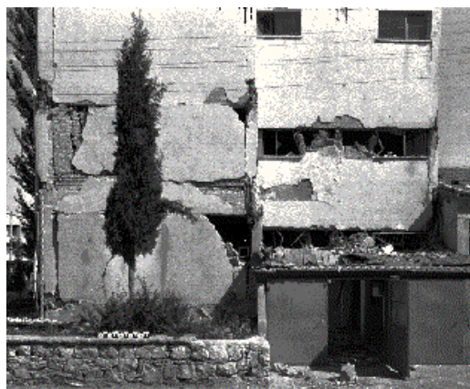
Figure 4-19: Detail Photo of Damaged Building (Volz, S.; 1997)
