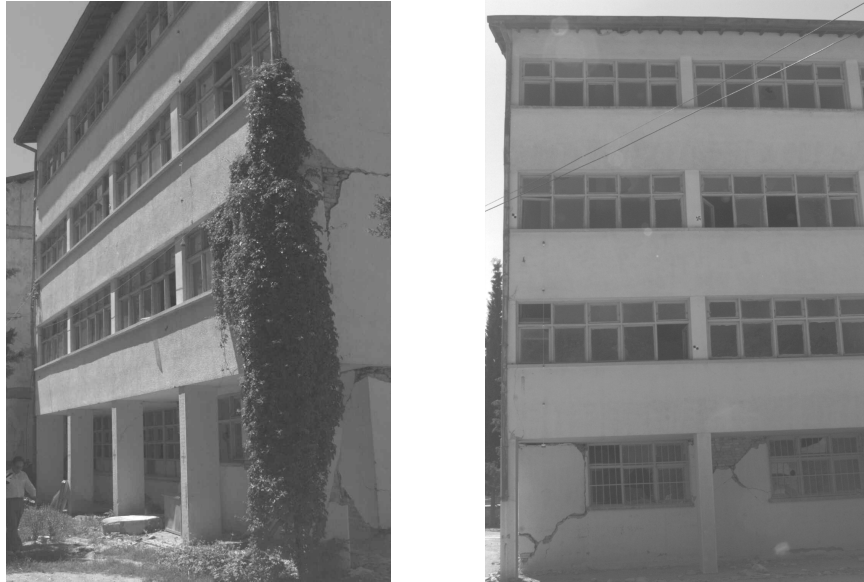
Figure 4-17: Digital Photo of Damaged Schoolhouse obtained by KODAK DCS 200 (Plumb lines for Scale and Verticality Information), Turkey (Altan, M. O. et alri; 1998, Streilein, A.; 1998)
