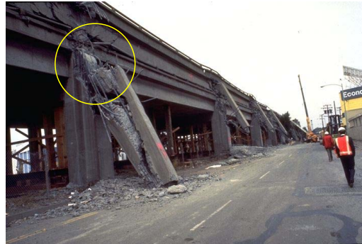
Figure 4-6: Loma Prieta, California earthquake in October 17, 1989 http://geohazards.cr.usgs.gov/eq/html/damage.html
