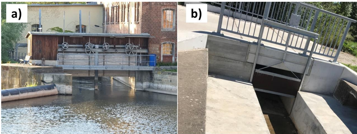
Figure 1: Application examples for sluice gates a) sluice gate in front of a former mill, now a hydroelectric power plant b) sluice gate for controlling irrigation ditches
