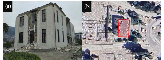
Fig. 11. Building with a damage grade of 4 on the EMS-98 scale in Antakya with damaged sides. Panel A is a photograph from the 13–17 March 2024 survey. Panel B is a MAXAR image on 8 February 2024 of the same building, with building footprints from the Microsoft dataset [26]. The footprint of the building is displayed in red. Despite being classified as “very heavy damage” in the field survey, the AI-based damage assessment computed the damage as 0%.
